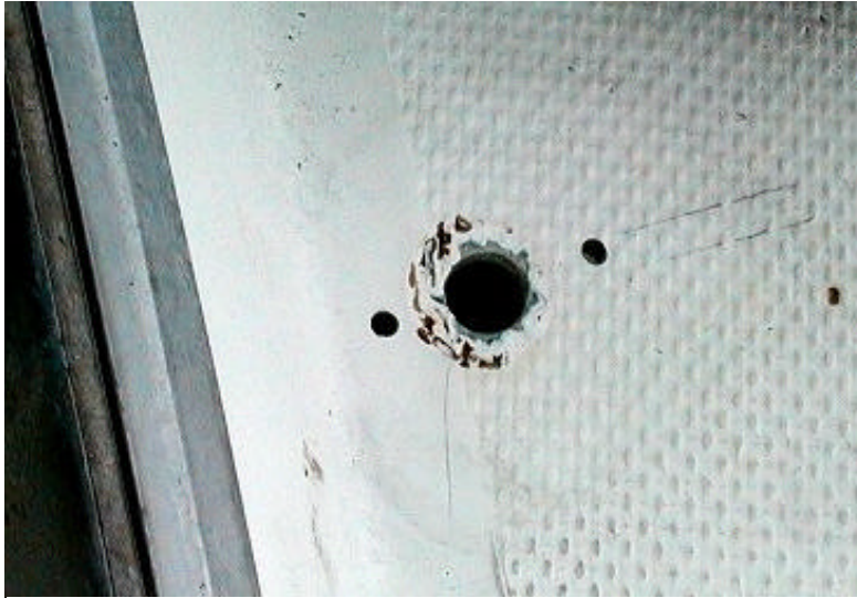
Figure 5 Old eyebolt removed. The hole has been enlarged to accept the new eyebolt and the two screw holes have been drilled through the deck and core using the new eyebolt as a template.
