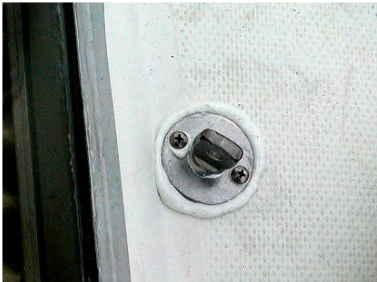
Figure 6 New eyebolt installed with 3M 4200 sealant squeezing out from beneath the flange. Cure time varies.
