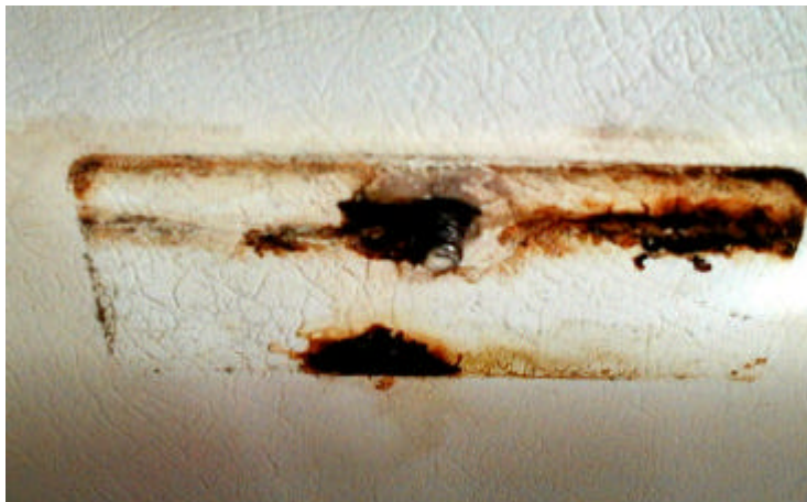
Figure 8 Rust stains left on cabin ceiling from old backing plate – clearly water had made it into the cabin and core at one time.
